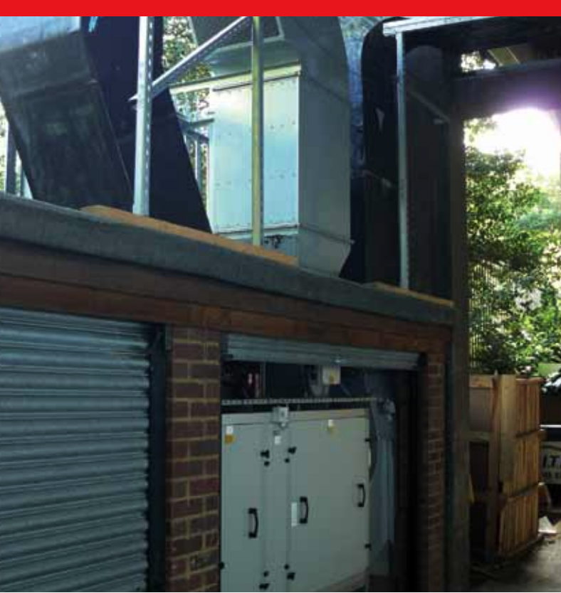
External plant room
