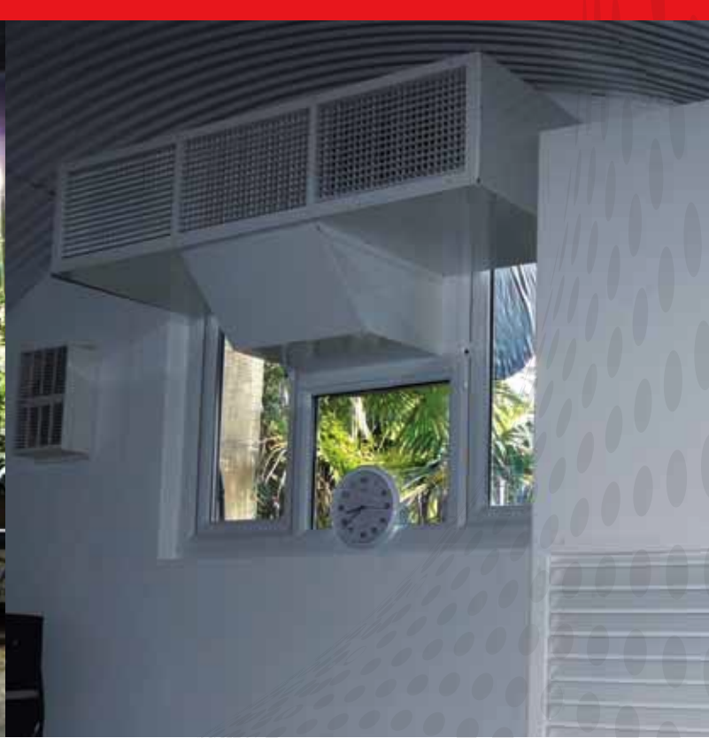
Pool hall supply and extract duct
